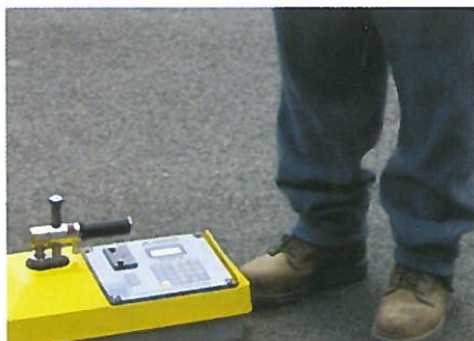
Nuclear Density Gauge to test the finished pavement to ensure proper compaction.
